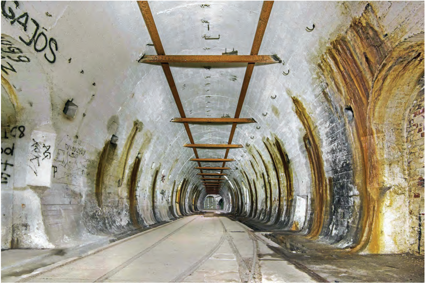
Part of the tunnel complex in the marshalling area near to shafts A1 to A3 in the massive MRU tunnel complex
